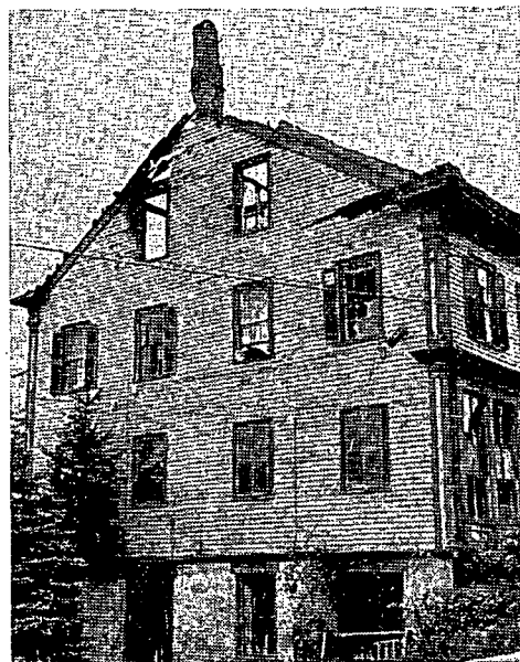
UPPER RIGHT window is where Rev. Buker dropped from. Caught on window blind on window just below.
